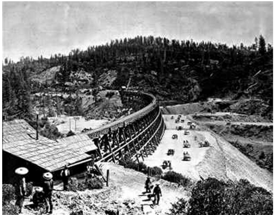
Chinese railroad workers transported dirt by the cartload to fill in this Secrettown Trestle in the Sierra Nevada Mountain.
